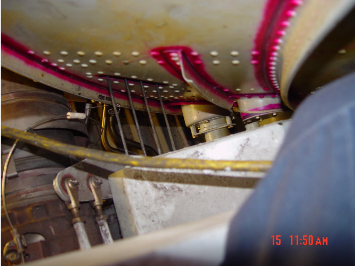
Figure 59. Pitch and yaw control cables pass through aft of pressure bulkhead looking down.
