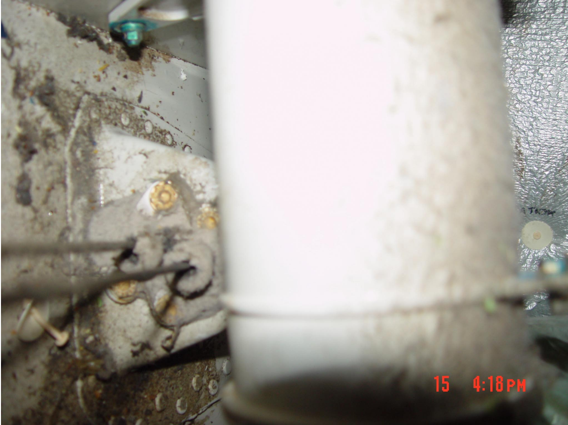
Figure 47. Roll control cables looking outboard and down near frame C47. Cables pass into wheel well.
