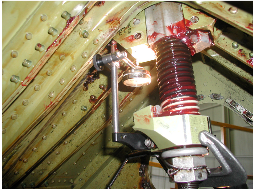
17. Close-up view of a typical dial indicator set-up for endplay checks performed at Tulsa. Note close proximity of mounting hardware to structure, orientation of the dial indicator face, size of the access hole, and the attachment of the C-clamp to the lower stop.
