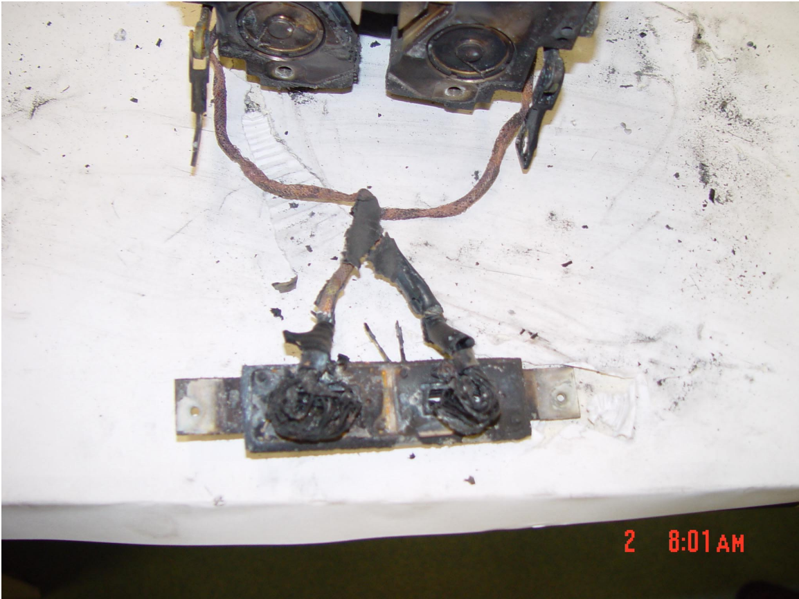
Figure 6. Detection Box Wiring.
