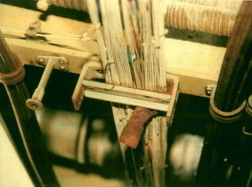
Systems 9 - 747-SL-20-048 - Fig. 4. Degraded raceway clamp cushion. The degraded portion of the clamp should be replaced to avoid subsequent damage.
