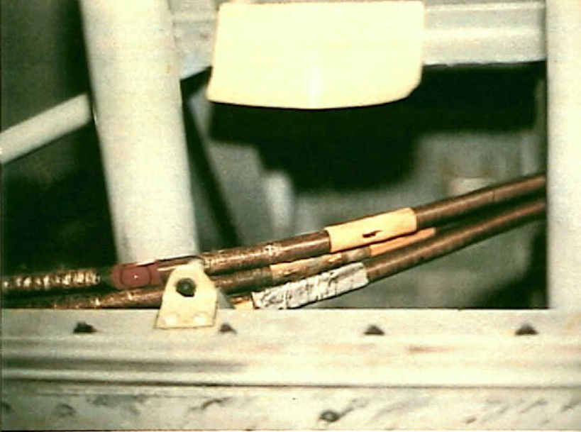
Systems 9 - 747-SL-20-048 - Fig. 36. Power feeders chafing at clamping points.
