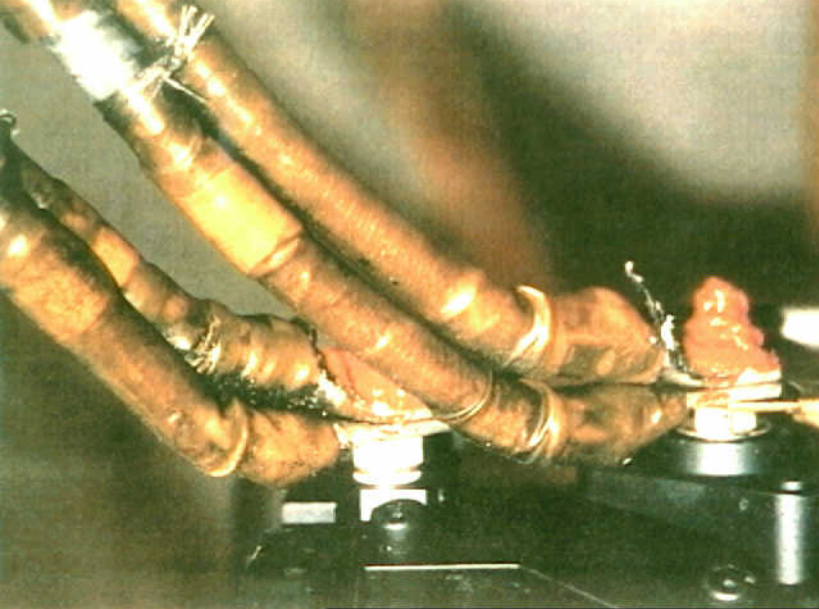
Systems 9 - 747-SL-20-048 - Fig. 33. Power feeder terminations in good condition. Terminations should be inspected for signs of over-heating.
