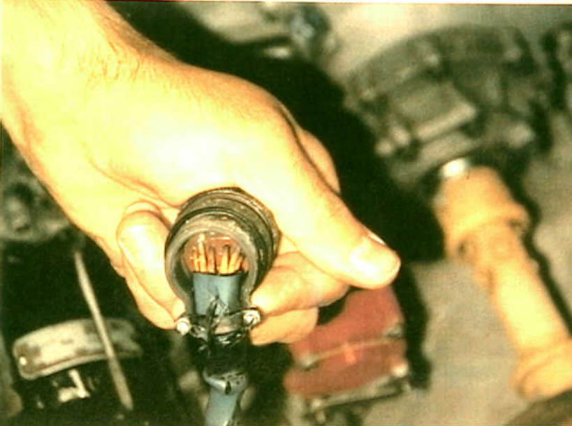
Systems 9 - 747-SL-20-048 - Fig. 20. Wing leading edge connector with lateral pressure due to missing backshell buildup and missing filler rods. This connector did have corrosion on the contacts.
