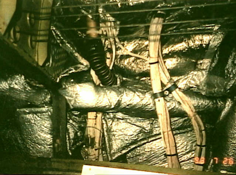
Systems 9 - 747-SL-20-048 - Fig. 14. This is a sidewall bundle with a large number of splices concentrated in one place.
