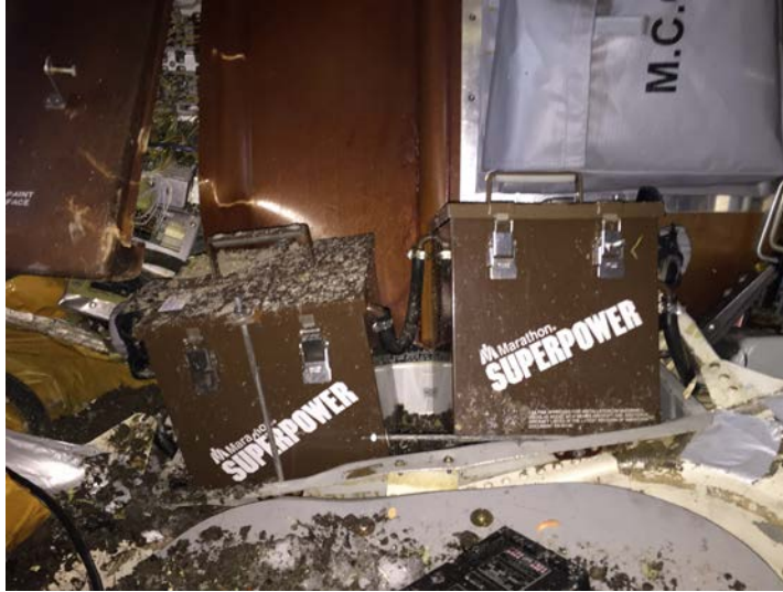
Figure 4 - Damage to Airplane Main Batteries and Shelf. The 110 Relay Panel is behind the batteries.
