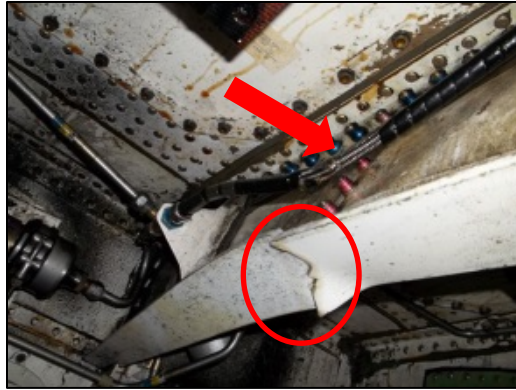
Figure 5 - The flexible hydraulic hose prior to removal. The fracture of the Nose Gear Retract Actuator Support Beam is circled; the abrasion on the flexible hydraulic hose is noted by the arrow.
