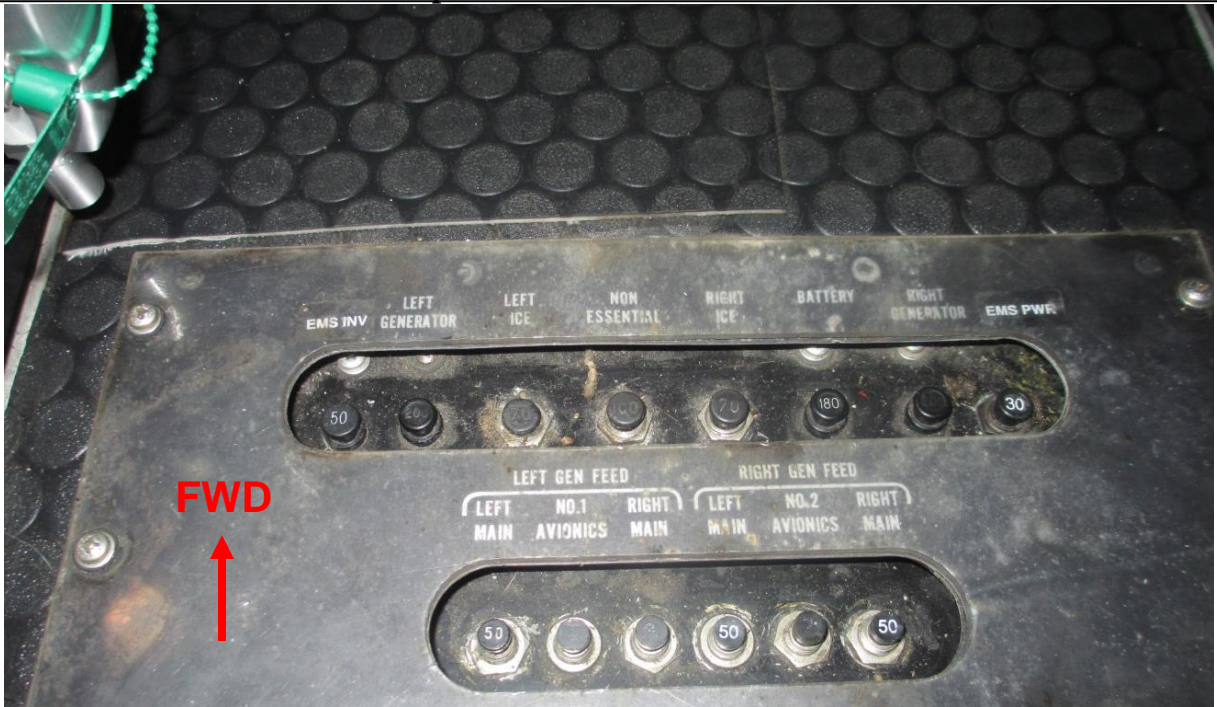
Figure 1 – Main bus tie circuit breaker panel
