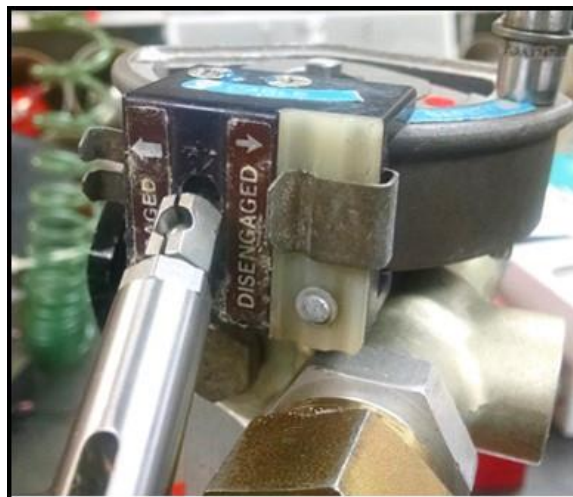
Photograph 12 - PFIM “ENGAGED” / “DISENGAGED” indication.
