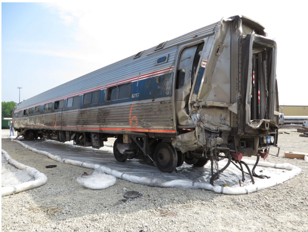
Figure 22. The right side of the sixth passenger car as viewed from the front of the car.
