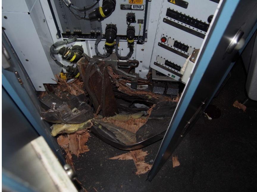
Figure 3- A view of a rail that punctured the floor of the car 7553
