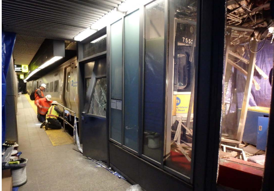
Figure 1- A view of the accident site
