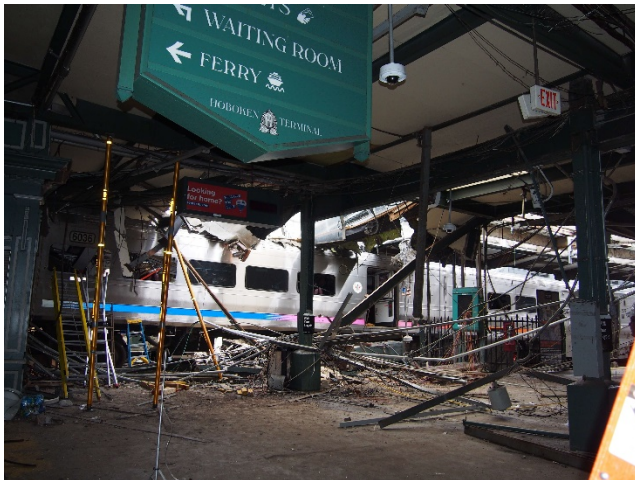
Figure 2- A view of the left side of the accident site and cab car
