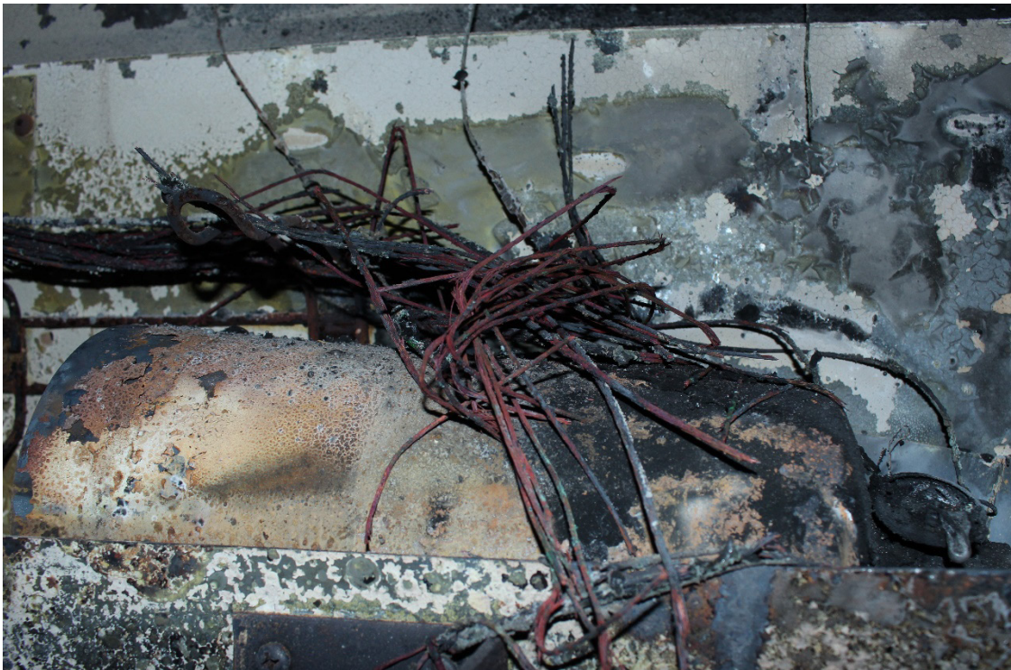
Photo #10: Close-up of fire damaged fire extinguisher in overhead compartment
