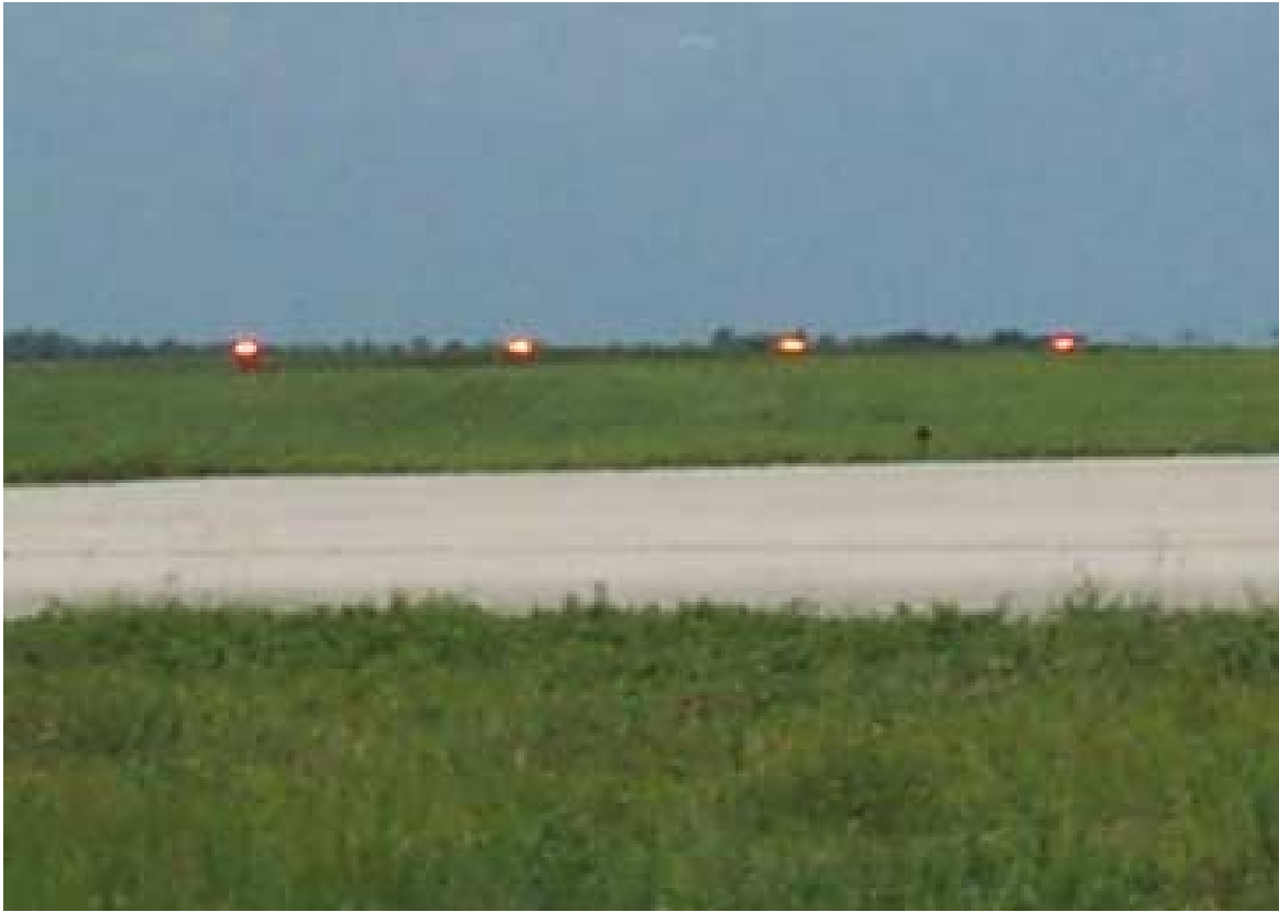
Photo 7: Four-unit ADB PAPI lighting system for runway 9, as viewed from taxiway 'M', looking east.
