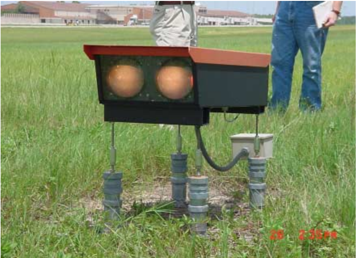
Photo 6: ADB Precision Approach Path Indicator (PAPI) Lighting Unit.
