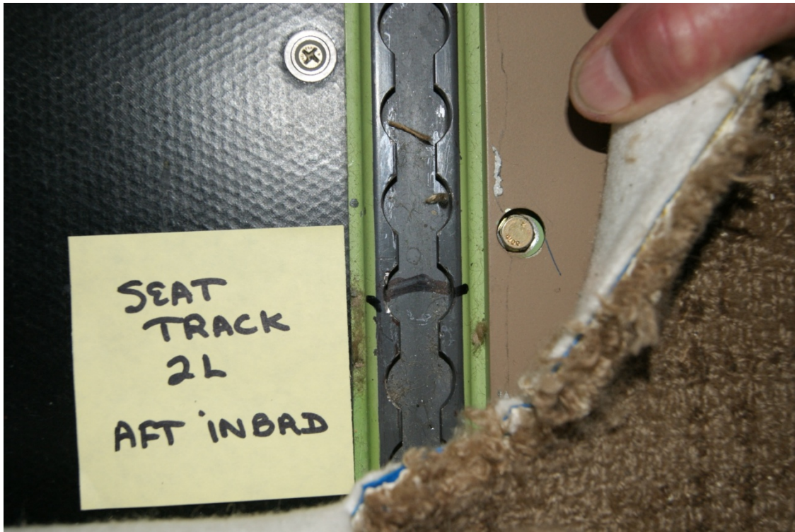
Photo 7: Seat L/H #2 aft inboard seat track.
