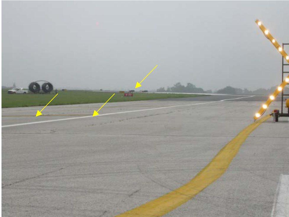
Photo 35. Runway 26 with the runway 4/22 intersection sign, lead-off line, white edge line, and yellow shoulder markings
