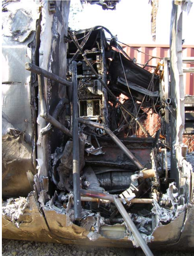
Photograph 9: Remains of MED after accident (Lancaster, TX).
