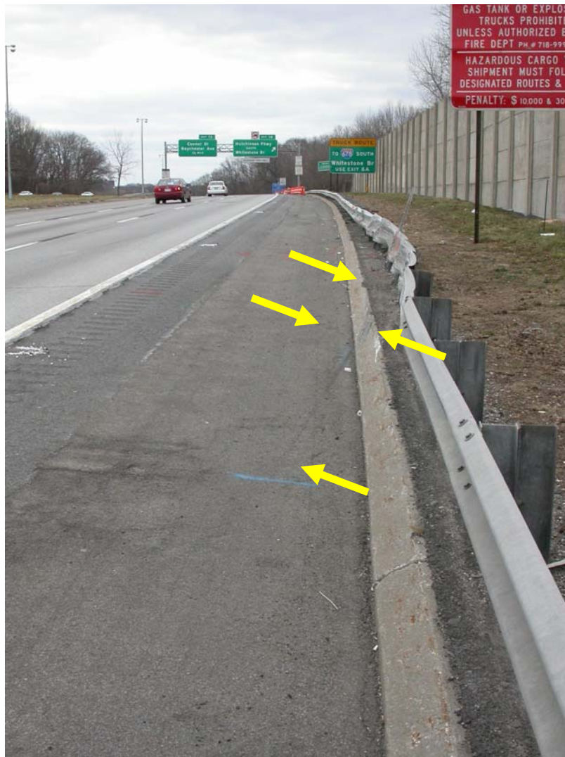
Figure 2 – Guardrail damage caused by the initial impact of the bus with the guardrail. Arrows point to tiremarks and scrapmarks indicating the path of the accident vehicle as it traveled across the 10 foot shoulder and impacted the guardrail. It could not be determined if the bus made contact with the red sign in the foreground. (Unless indicated by an arrow, tiremarks and scrapmarks shown in the photograph are not associated with this accident.)
