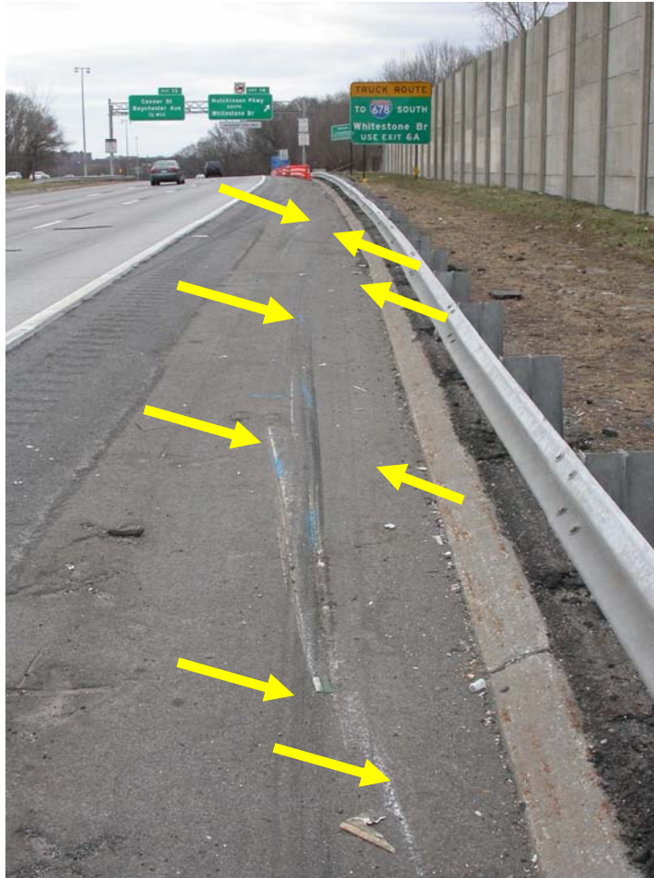
Figure 3 – After initially striking the guardrail the bus veered away from the guardrail and lost contact the guard rail for short distance. The arrows shown in the photograph indicate evidence of the path of the bus during the time it lost contact with the guardrail. Note that there is no evidence of contact damage from the bus visible on the guardrail. (Unless indicated by an arrow, tiremarks and scrapemarks shown in the photograph are not associated with this accident.)
