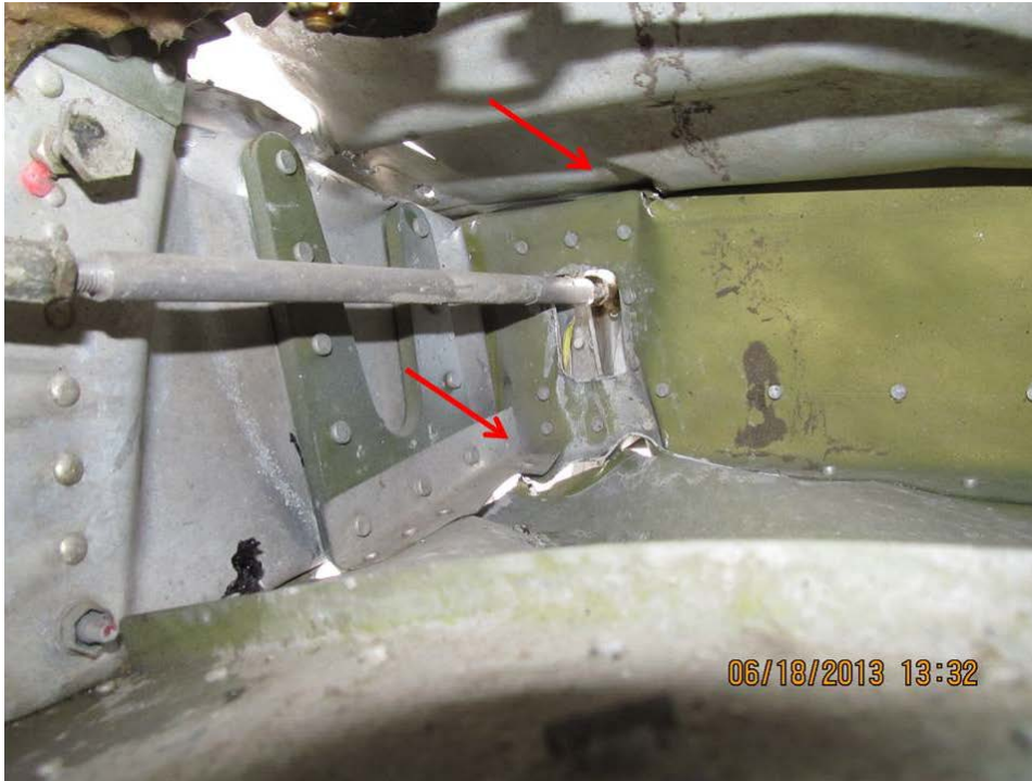
Photo 19 - Compression damage to top and bottom rear spar caps.
