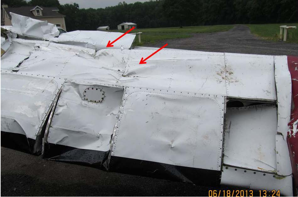
Photo 15 - One arrow highlights compression damage on the upper cap of the rear spar. The other arrow highlights a major wrinkle across the top of the right wing.
