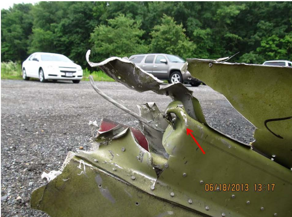
Photo 10 - Top cap of rear spar buckled in compression.
