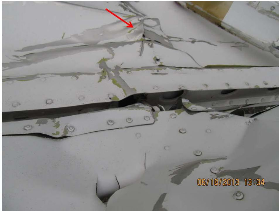
Photo 22 - Compression damage of upper cap of rear spar.
