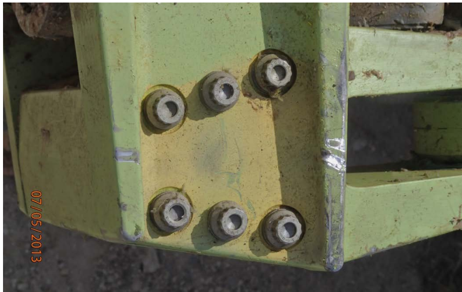
Figure 71 - Jack Screw Collar Fitting Witness Mark Close-up
