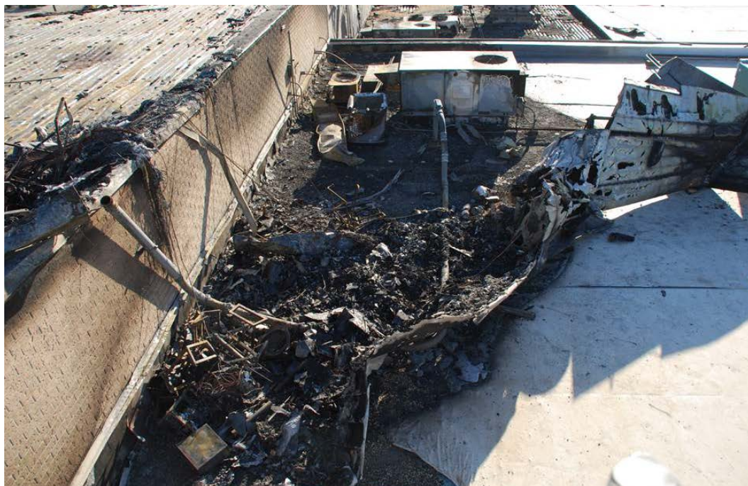
Photo 6 – Cabin top is inverted, vertical tail and rudder to the right on 2 nd roof level
