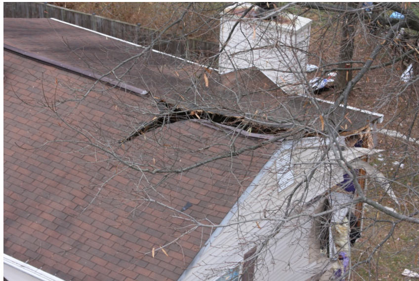
Figure 7. Cut in roof of 19740 Drop Forge Lane.
