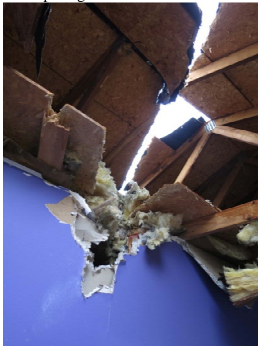
Figure 8. Initial contact of roof and interior bedroom wall inside 19740 Drop Forge Lane. This view is back toward the flight approaching the house, aligning the two contact points.
