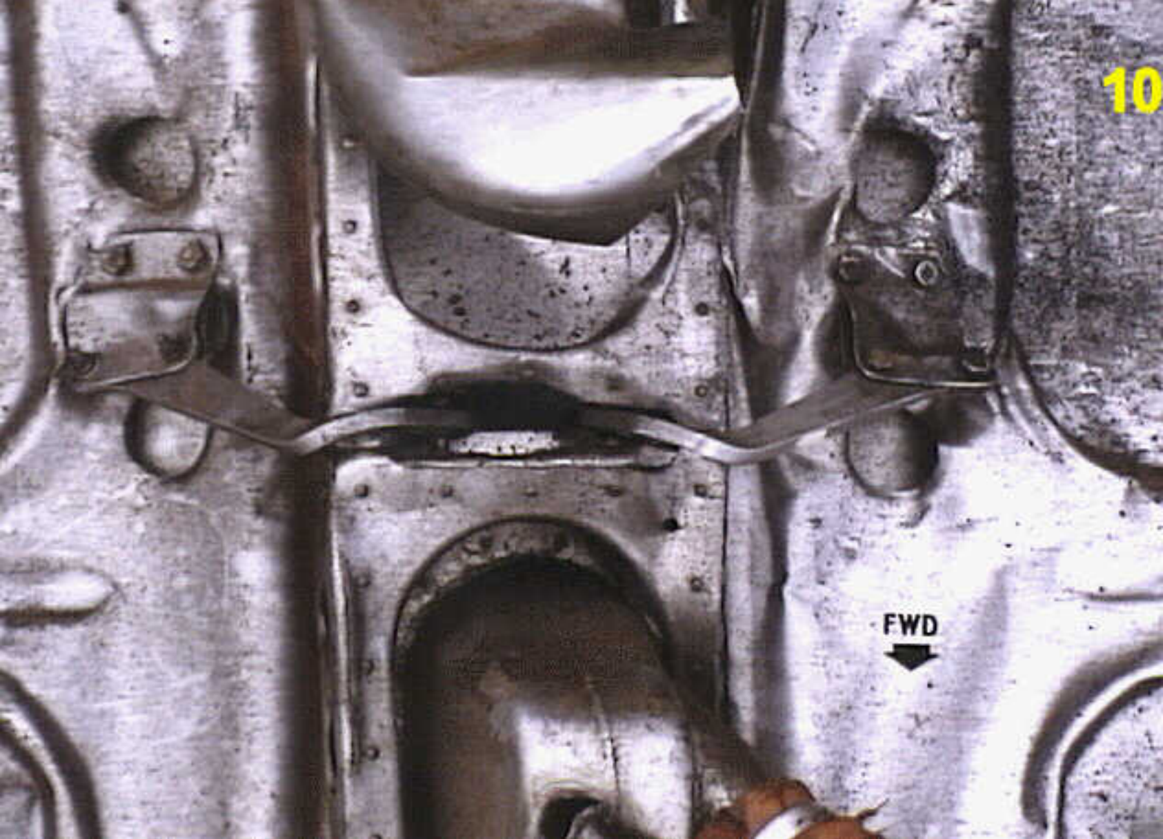
Structures 7A - Photo 10. Damage to middle hinges of left forward cowling doors.
