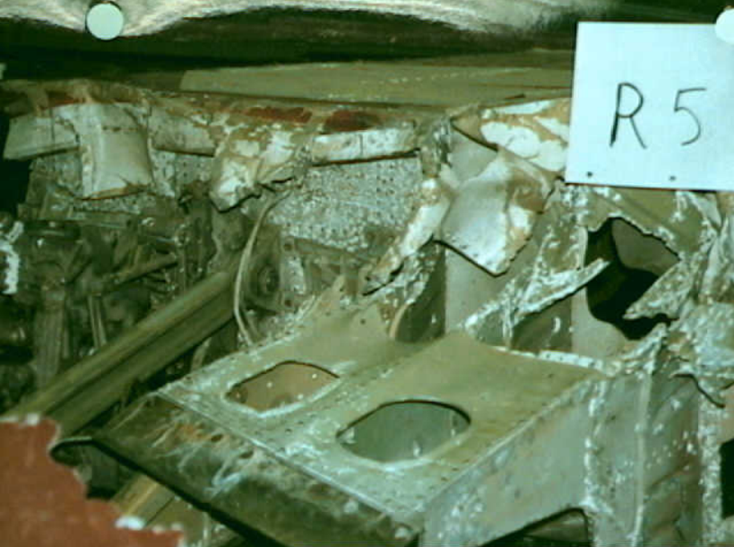
Structures 7 - R-5 Photo 1
