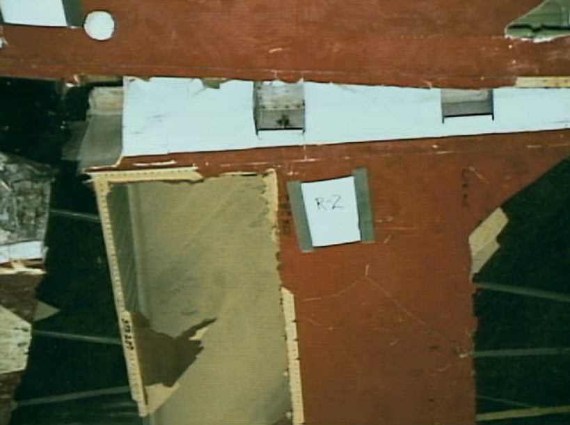
Structures 7 - R-2 Photo 2
