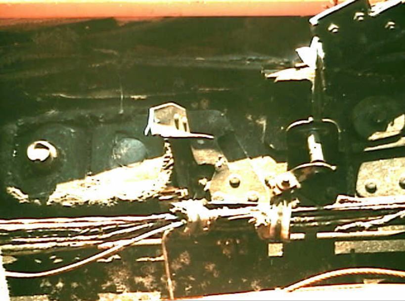
Structures 7 - Photo. 9 - View of the outboard attach fitting upper fasteners for the outboard flap hinge. Note the tension fracture of the inboard bolt (on the left).
