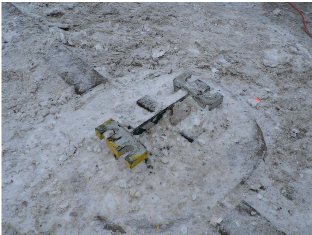
Figure 7. Base of vertical fence support, showing slots that the mounting bolts can be driven from in an impact. (For orientation, the runway is toward the lower left and street is to upper right.)
