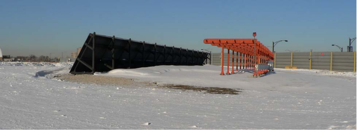
Figure 15. Opposite end of the runway, located at the southeast corner of the airport, showing a similar installation of the blast fence, instrument landing system array, and in background is the frangible perimeter fence, using I-beam vertical supports and stacked lightweight acoustic panels.
