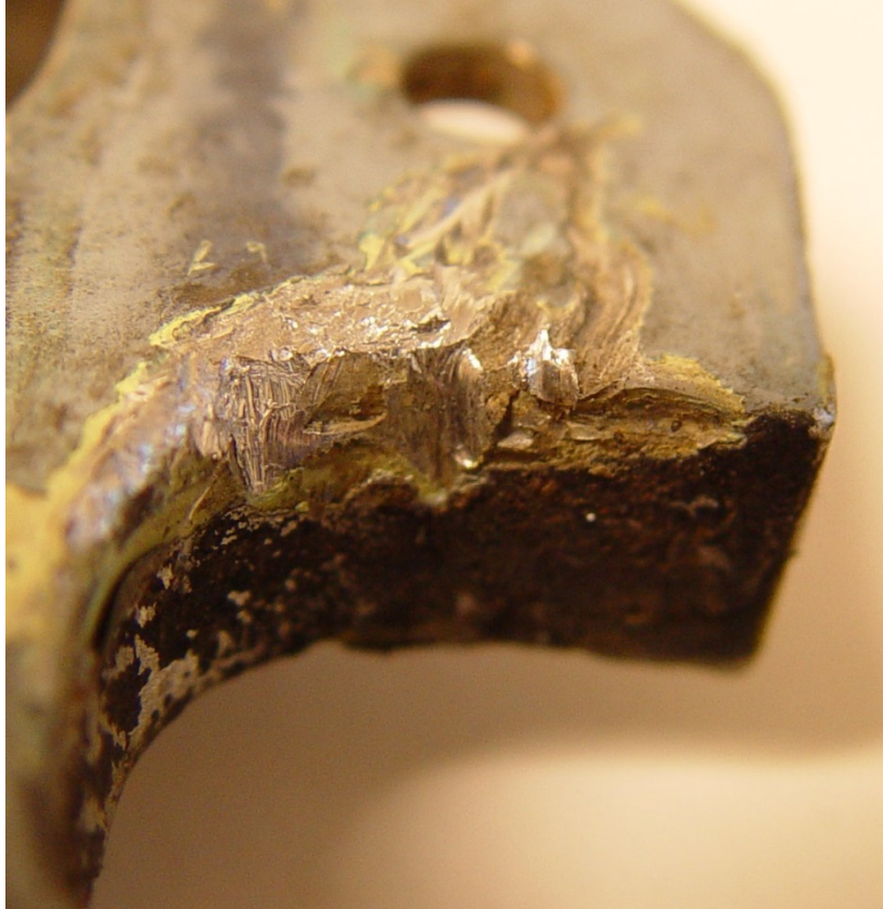
Figure 23 - Damage to upper, aft edge of right, lower stabilizer fitting
