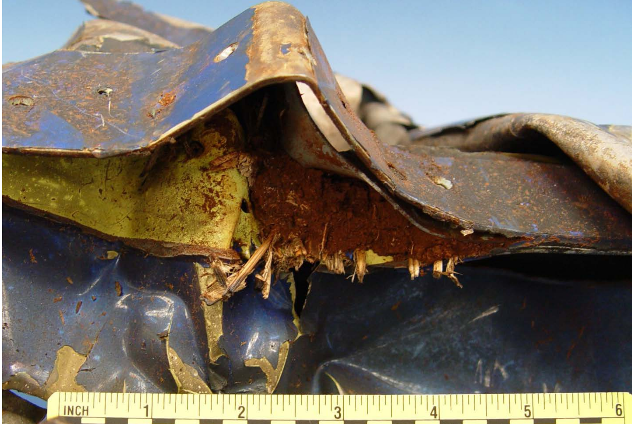
Figure 9 – Dirt and wood debris between right spar and spar strap
