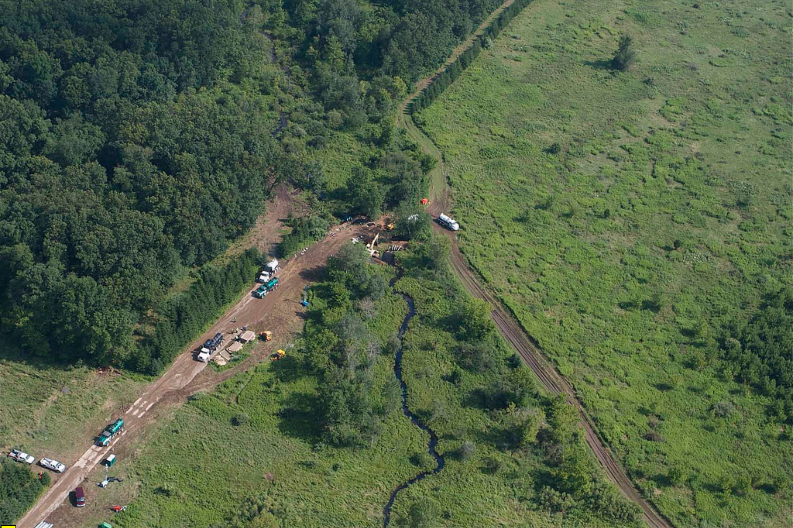
Site of MI Aerial View of Talmadge Creek Near Pipeline Rupture, July 28, 2010
