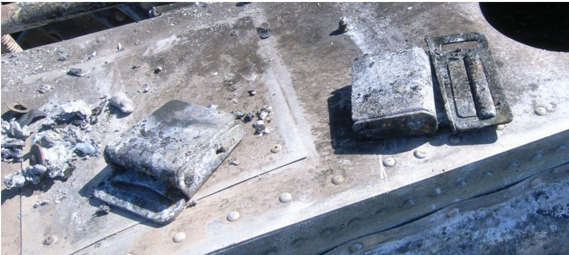
Figure 11 - Buckled Lab Belt Latch
