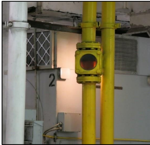
Figure 12. Bull's-eye for monitoring lube oil flow from gravity tank. (Photo from El Yunque )
