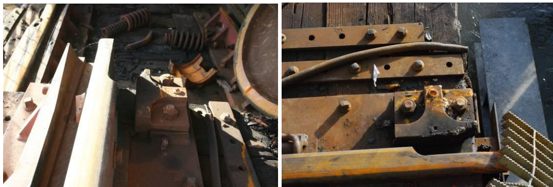
Figure 4. North End Proximity Switch Back View (L) and Overhead View (R).
