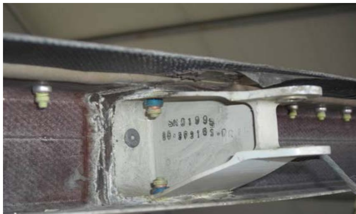
Fig.1 – Corroded center fitting without aluminum bonding strips
