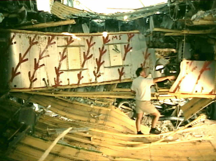
Sequencing Group 18 - Appendix B - Photo 13. View showing damage to mid spar.
