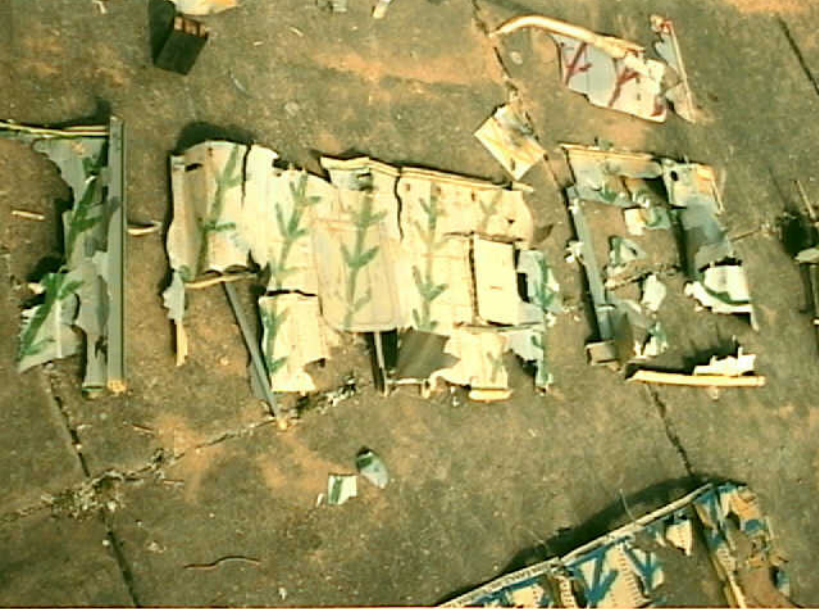
Sequencing Group 18 - Appendix B - Photo 12. View showing deformation & damage to SWB#2.
