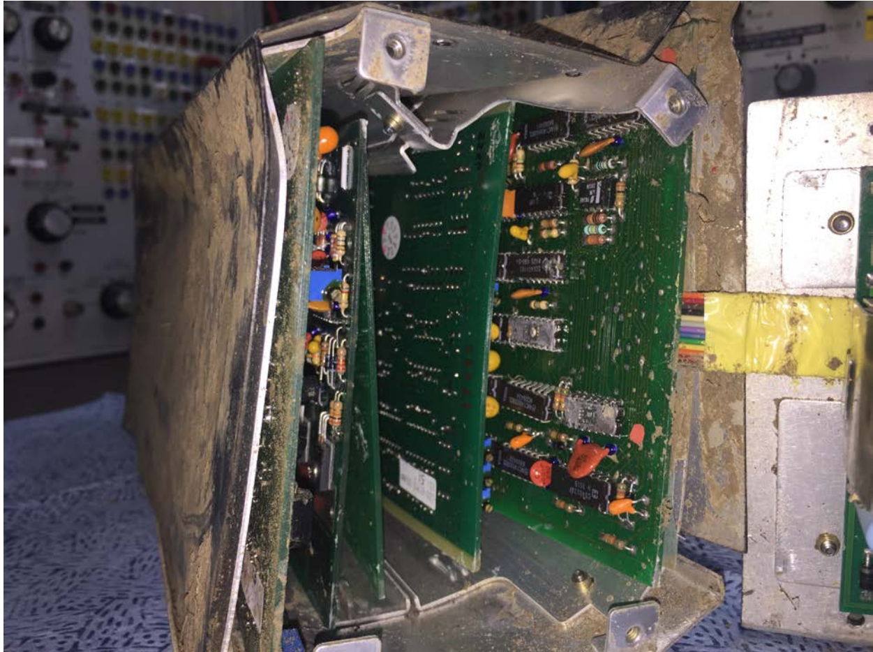
Internal view of KC 295 with end plate containing the power supply removed. Several damaged electrical components can be observed.
