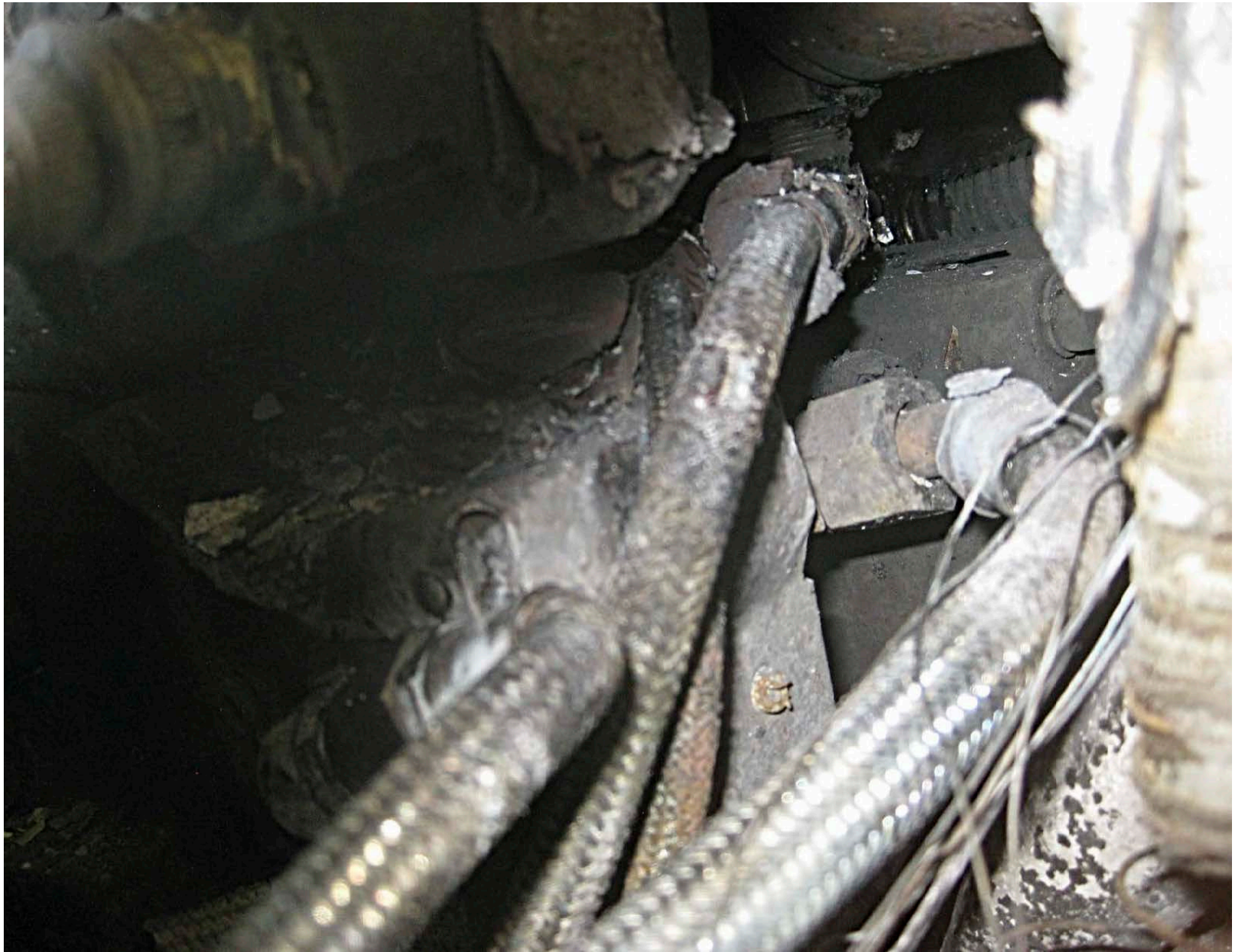
Photo 14 - Fuel lines going into and out of the fuel pump.
