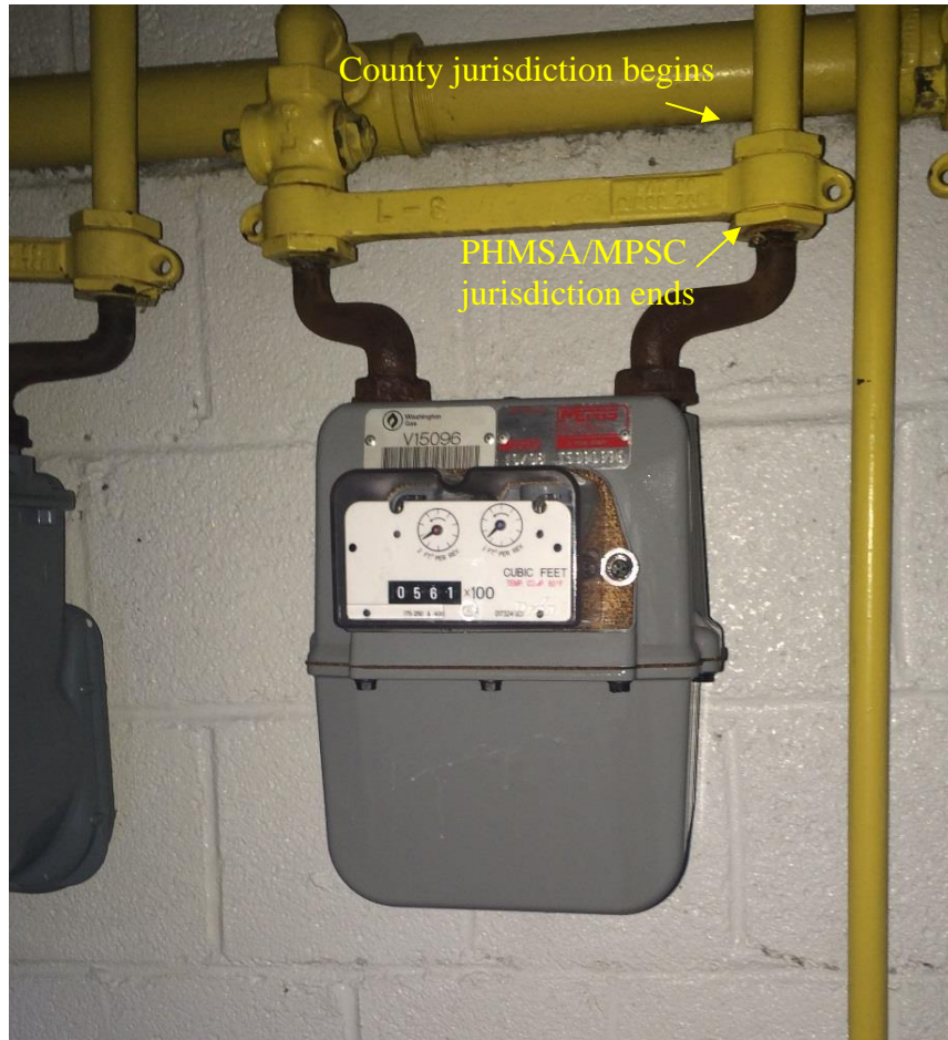
Figure 1: Exemplar Gas Meter in Flower Branch Apartment Complex
