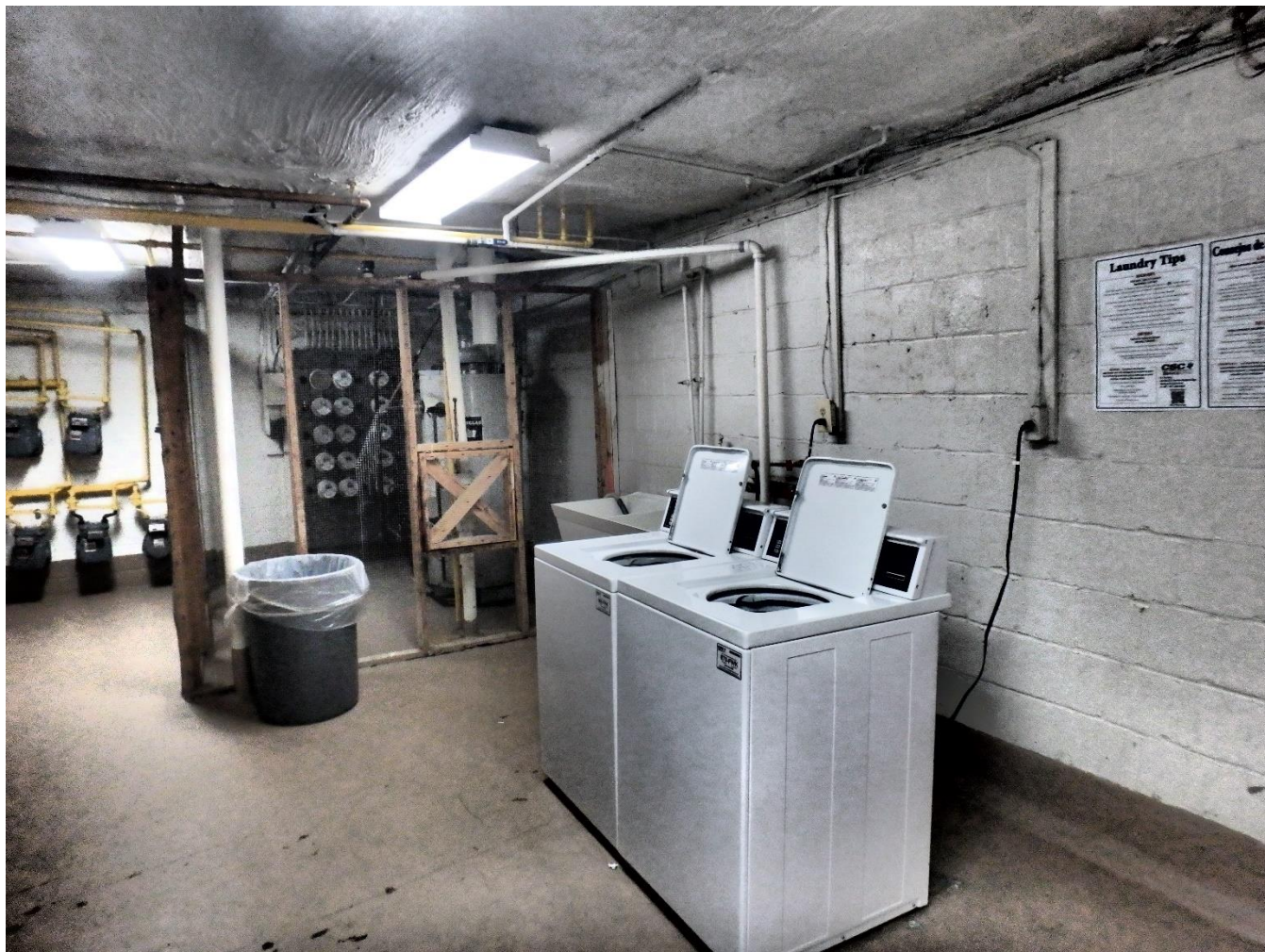
Figure 3: Exemplar Gas Meter room in the Flower Branch Apartment Complex
