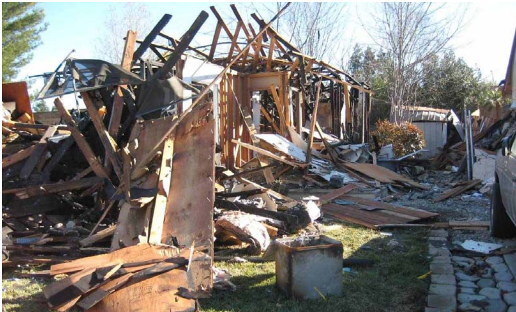
FIGURE 1 – DAMAGE CAUSED BY THE EXPLOSION
