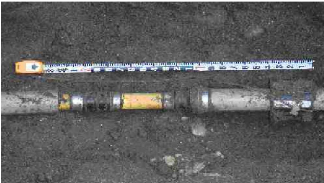
FIGURE 2 –LEAK AS DISCOVERED IN THE FIELD. THE “SPOOL PIECE” IS IN THE CENTER OF THE PHOTOGRAPH AND THE LEAK IS ON THE RIGHT SIDE OF THE 1¼-INCH COUPLING.
