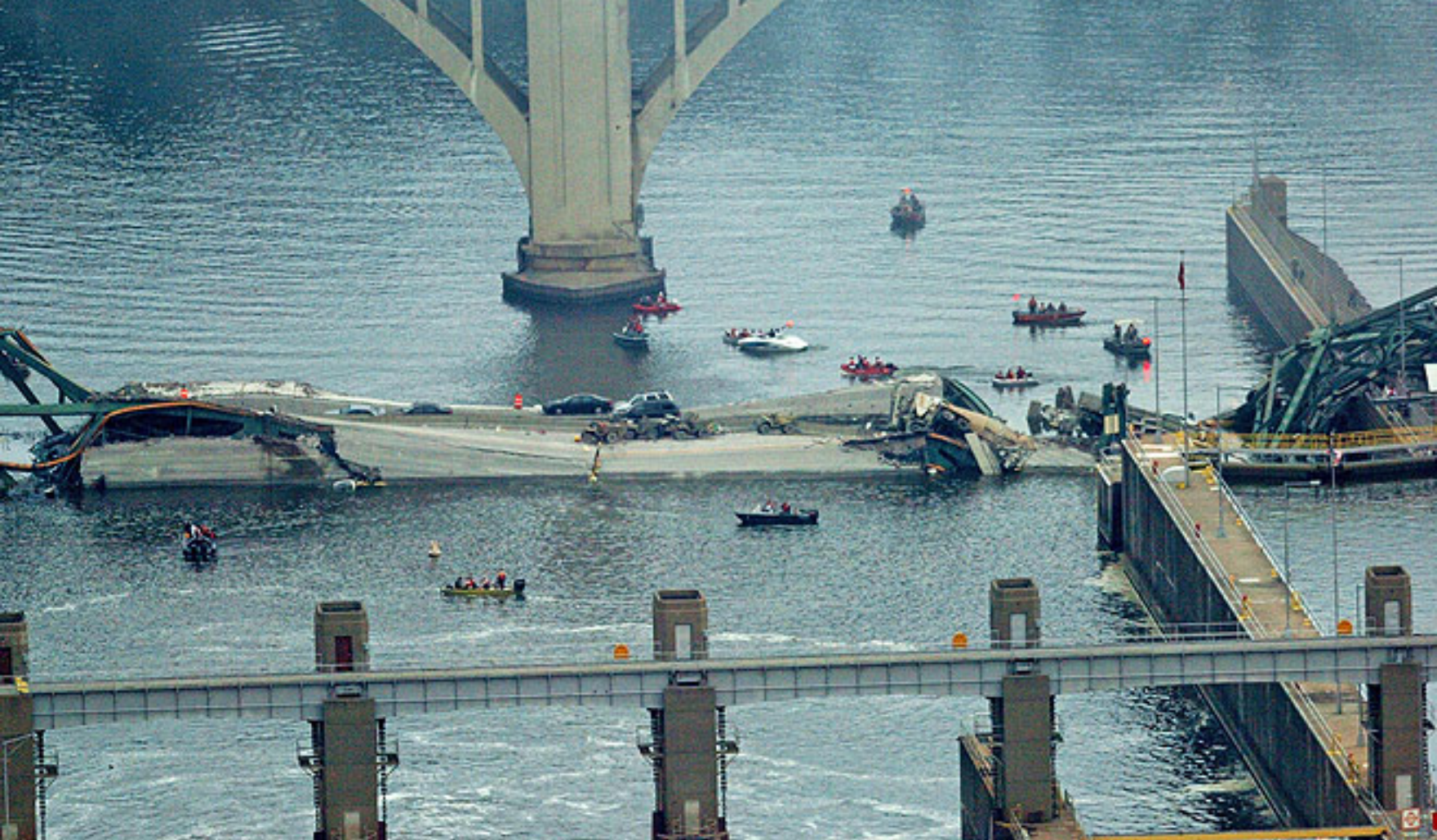
Presentation 11 - Photo of post-collapse rescue efforts (source MPD)
