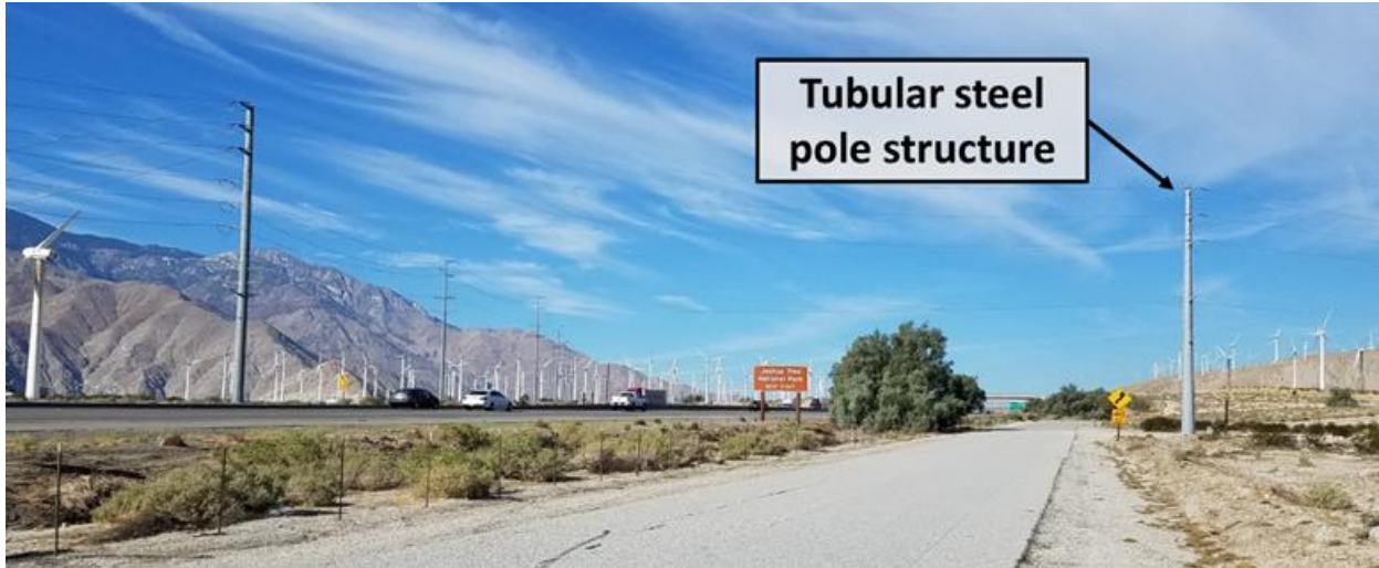
Figure 2. Westbound view of the new tubular steel pole structure at the intersection of the northwest corner of 20th Avenue and Diablo Road.
