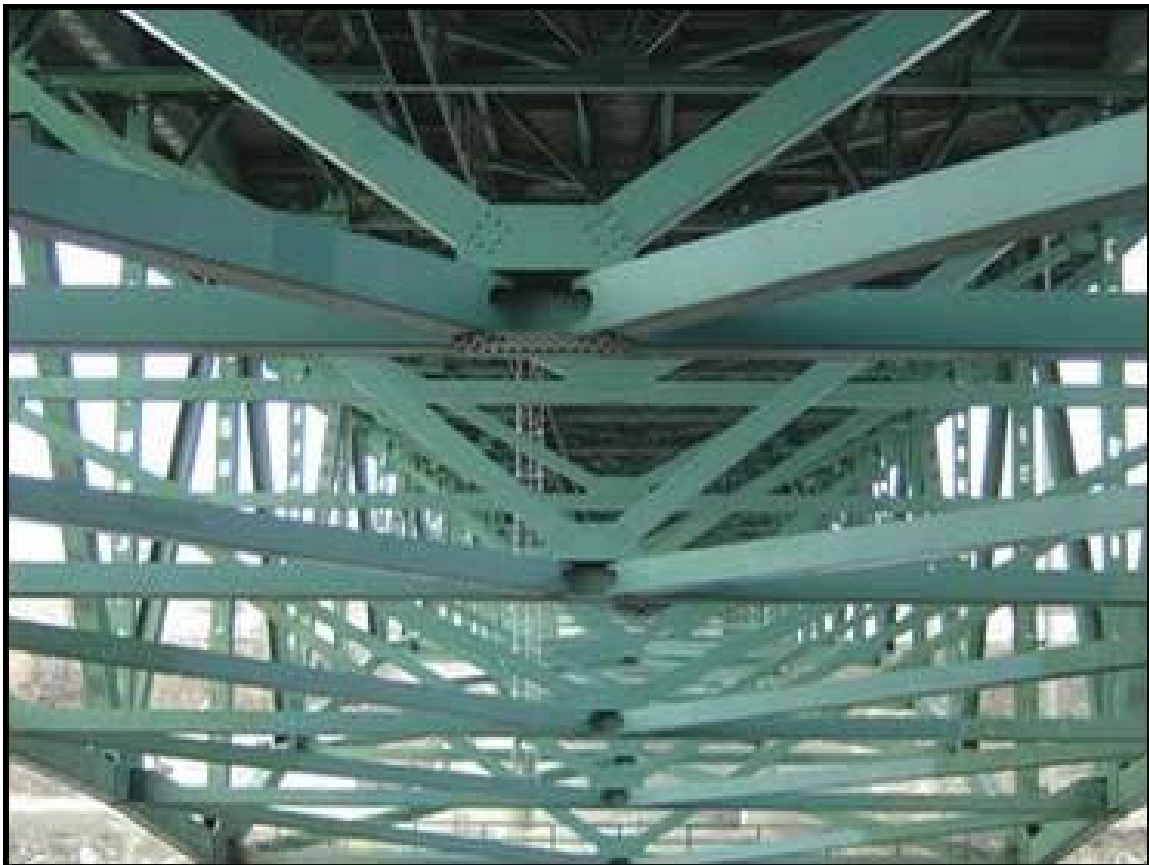
Overviews (from below of the bridge showing lateral and sway braces), Source University of Minnesota, 8.jpg
