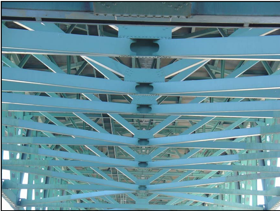
Overviews (from below of the bridge showing lateral and sway braces), Source Individual, DSC07297.JPG
