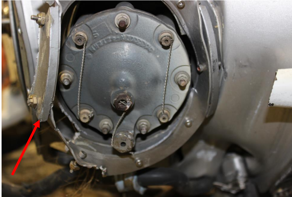
Photo No. 78, view of the right hand valve
