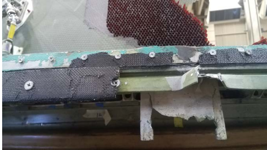
Photo No. 16: View of the upper aft bulkhead's outer stiffener was torn and deformed. (Boeing)
