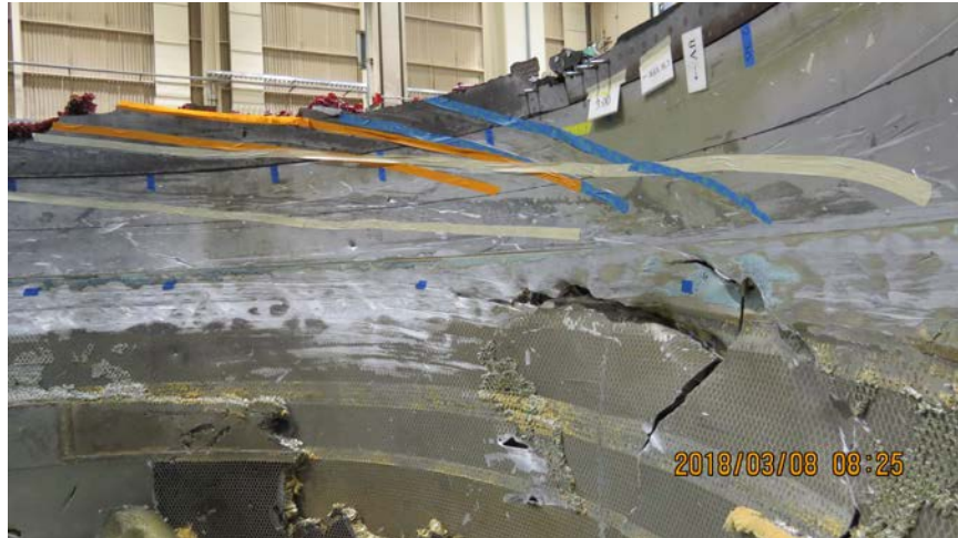
Photo No. 33: View of inside of the fan case showing the three tracks that spiral across the fan case onto the inlet duct. (P&W)
