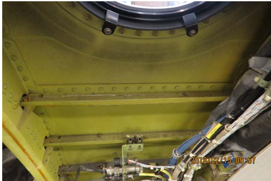
Photo No. 58: View of top of bent and cracked zee stringer at BSTA 913. (P&W)
