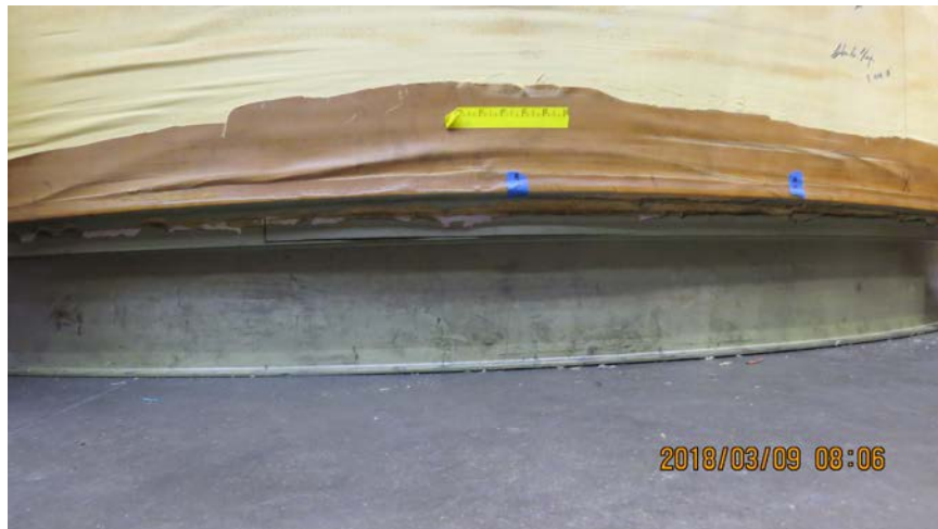
Photo No. 27: View of aft edge of the Kevlar wrap showing the crack in the epoxy. (P&W)
