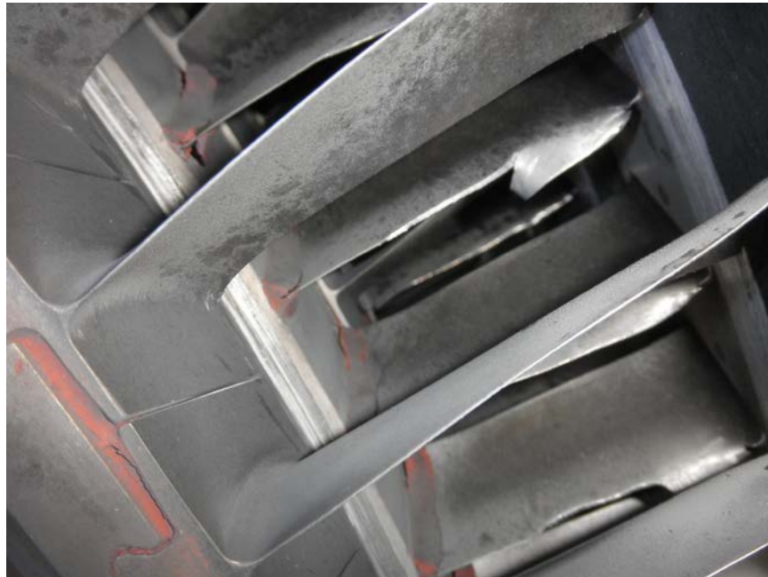
Photo No. 40: Close up of 3rd and 4th stage compressor blades and 3rd stage compressor vanes showing damage to the airfoils.
