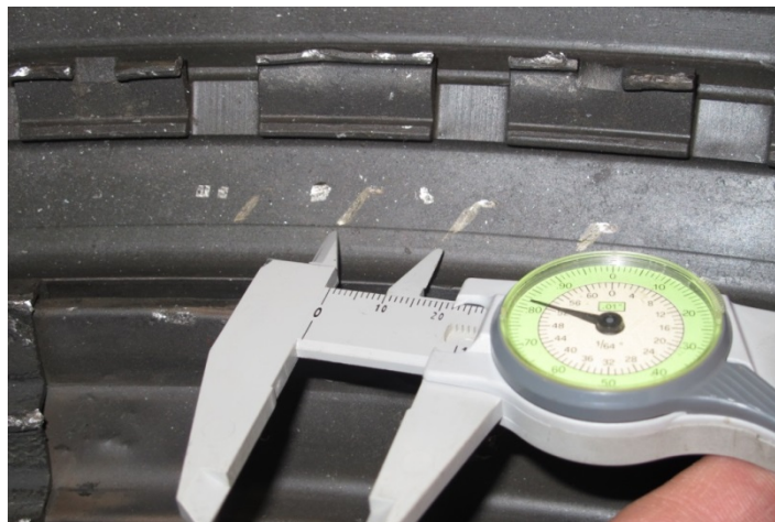
Photo 28- Impact Marks Along 3 rd Stage Vane Track, Vanes, and Heat Shield Missing
