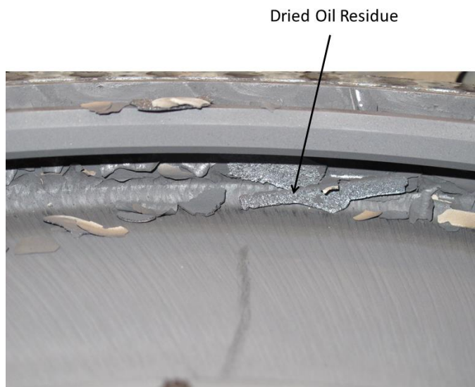
Photo 33- 1-to-2 Seal Oil Residue
