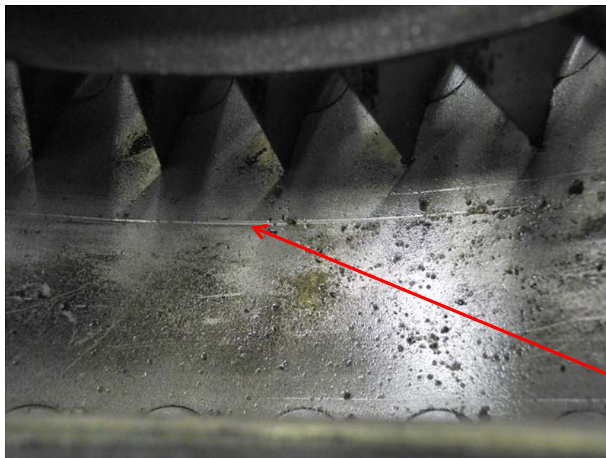
Figure 38 – 2 nd Stage Axial Compressor Shroud
