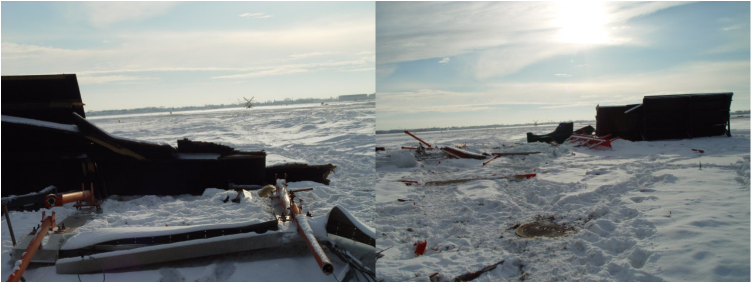
PHOTOS 3 AND 4: DAMAGED WOODEN BLAST FENCE AT THE DEPARTURE END OF 31C
