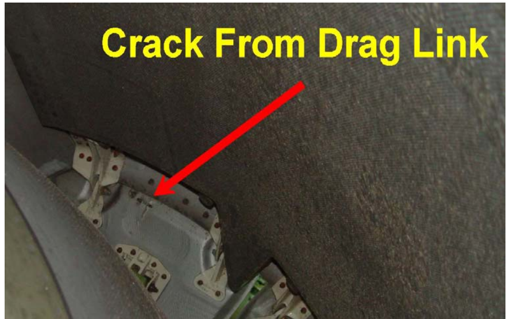
PHOTO 18: CRACKED BLOCKER DOOR
