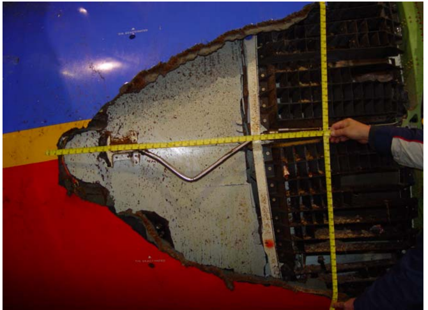
PHOTO 17: BENT ACTUATOR PUSH/PULL ROD
